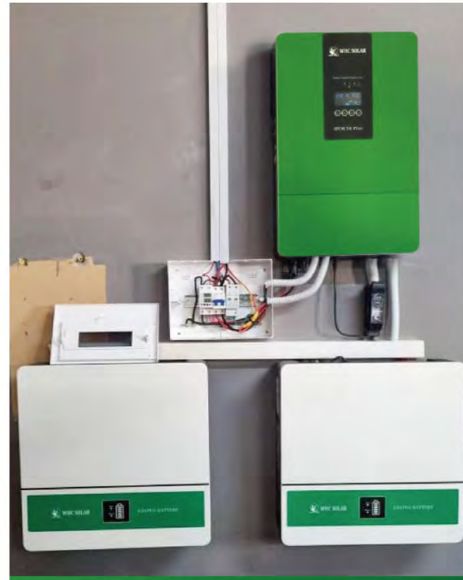
WHC-5KW-Li-10KWH Solar Energy Storage System Location: Lusaka, Zambia
