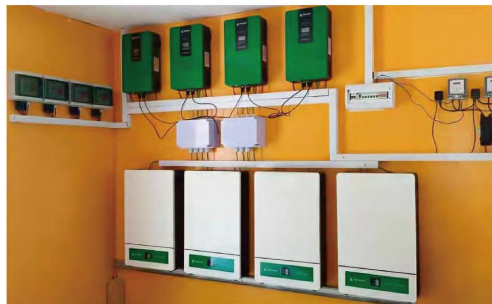
WHC-20KW-Li-40KWH Solar Energy Storage System Location: Dakar, Senegal
