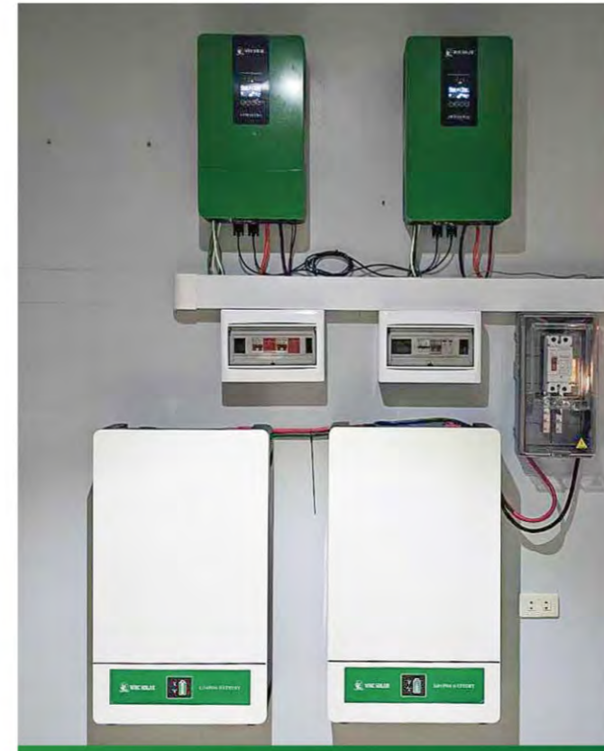
WHC-10KW-Li-20KWH Solar Energy Storage System Location: Manila, Philippines
