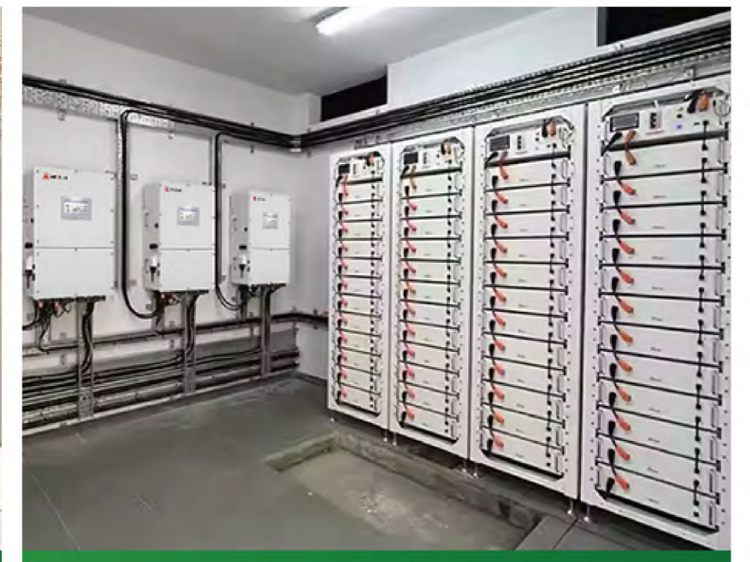
WHC-150KW-Li-430KWH Solar Energy Storage System Location: Johannesburg, South Africa
