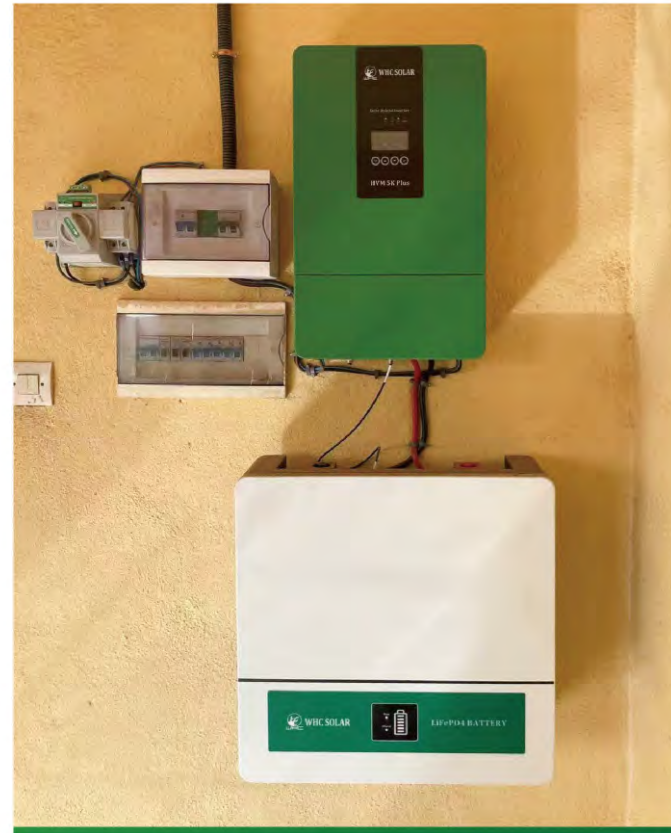
WHC-5KW-Li-5KWH Solar Energy Storage System Location: Bamako, Mali
