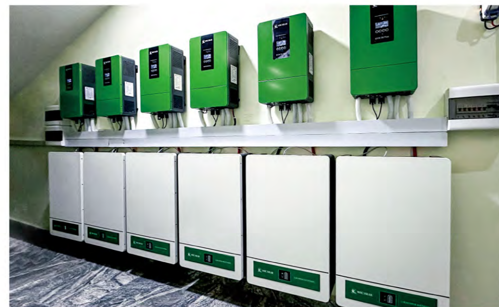
WHC-30KW-Li-60KWH Solar Energy Storage System Location: Kano, Nigeria
