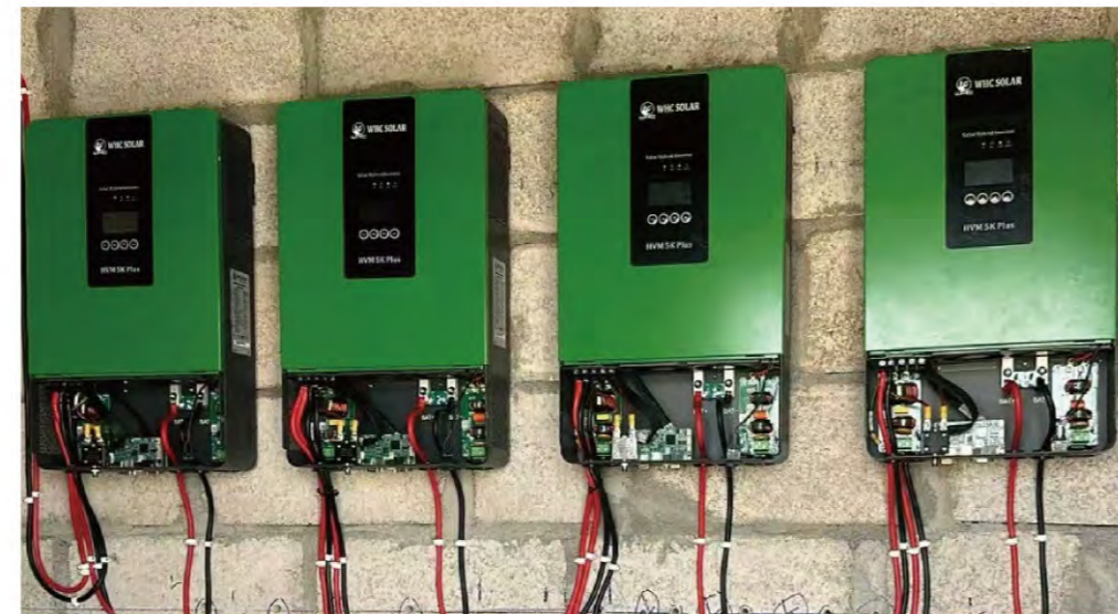
WHC-20KW-Li-30KWH Solar Energy Storage System Location: Dubai, UAE
