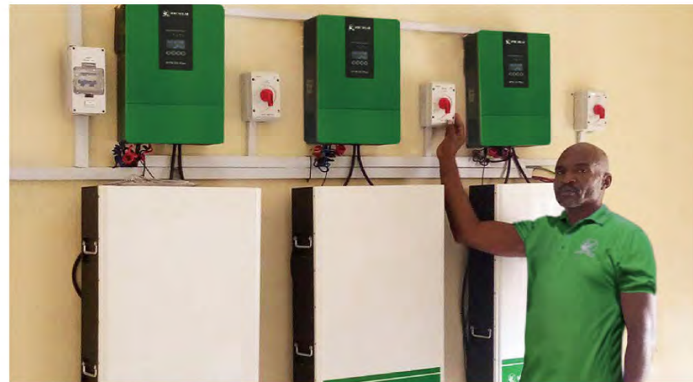
WHC-15KW-Li-30KWH Solar Energy Storage System Location: Freetown, Sierra Leone
